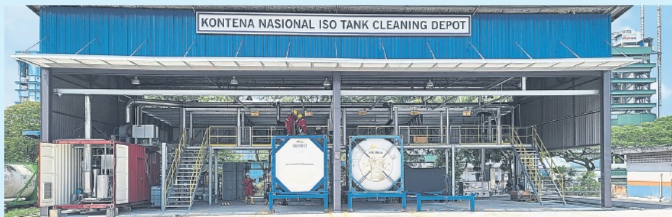
The first of its kind in Malaysia, the ISO Tank Cleaning Depot uses a comprehensive cleaning ecosystem from Groninger Cleaning System
